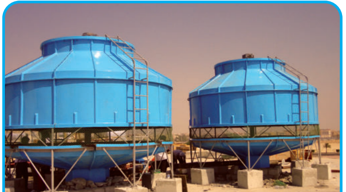
Cooling Tower at BGB
