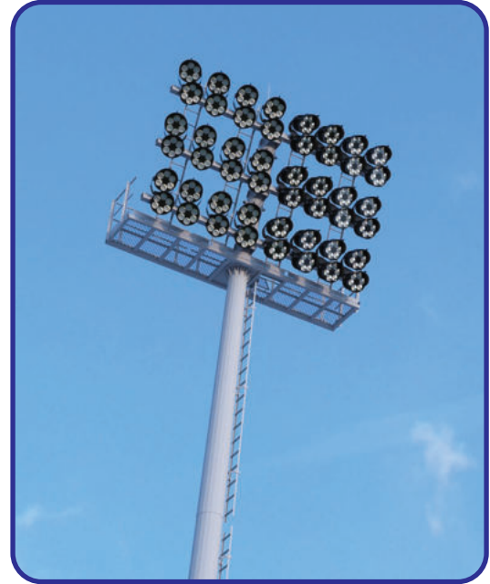
Stadium Light Tower
