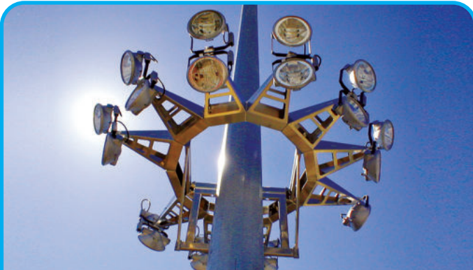
Flood Light Tower/ Highmast at Chittagong
