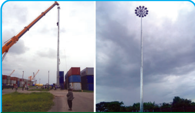
Mongla Port High Mast Lighting
