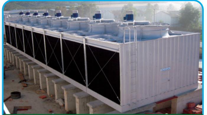
Ocean Cooling Tower at Biman & BAT
